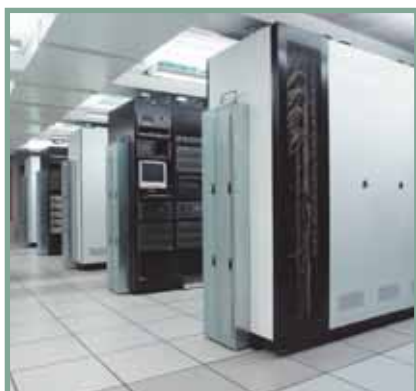
Data centre cooling
